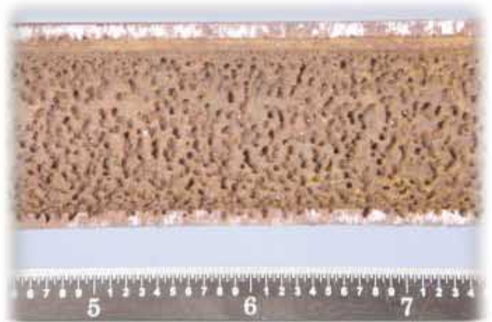
Example of Localized Corrosion (Pitting)
